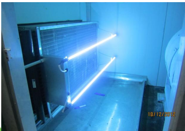
One of the UVC sterilisation systems installed at Council's head office
